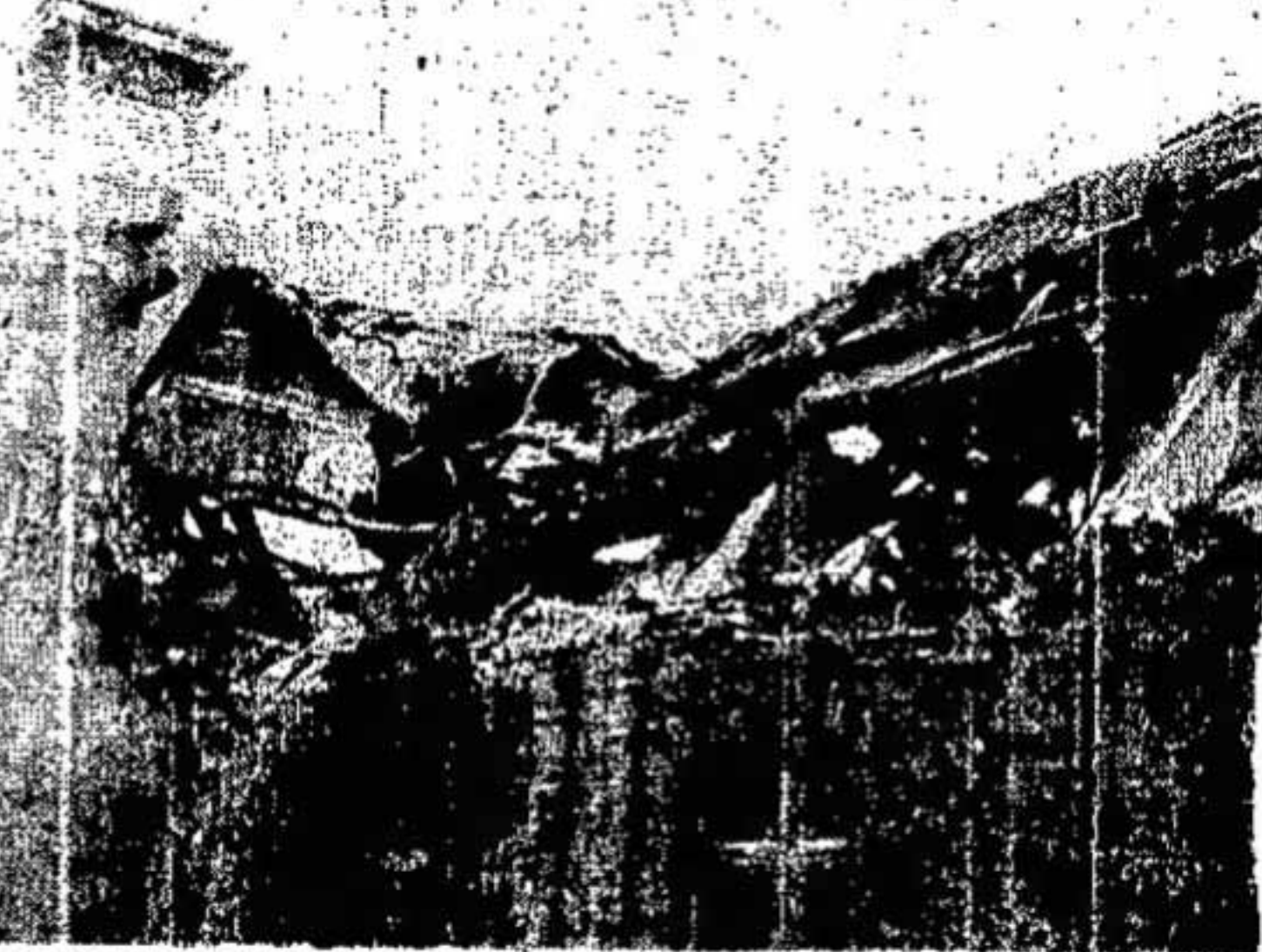
TWISTED STEEL —Steel superstructure of the gymnasium roof can be seen in this picture, taken from a scoreboard platform. Intense heat of the fire is evidenced by the condition of the girders.
